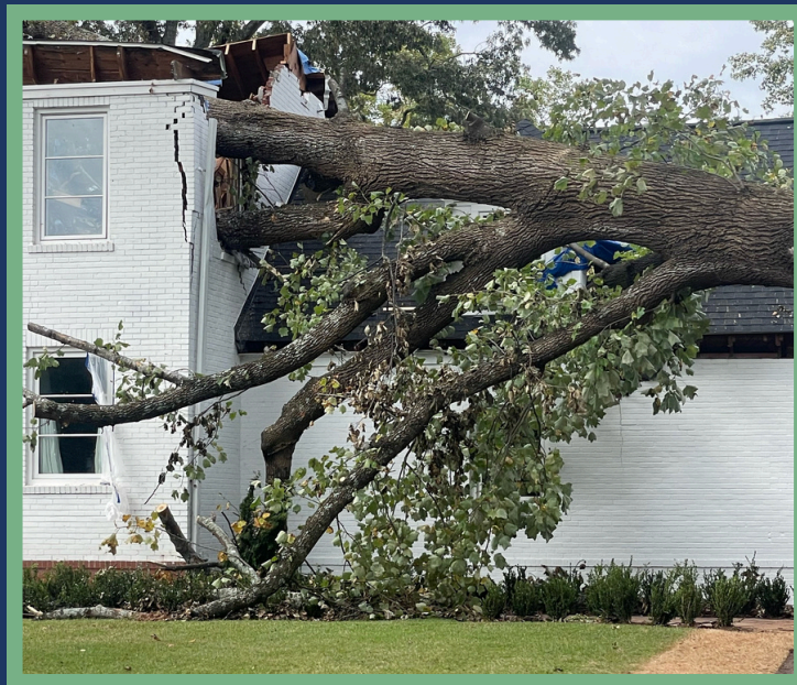
Tree damage to Greenville County residence
